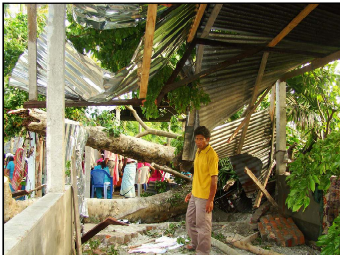
Building damage wrought by Cyclone Aila in early June
